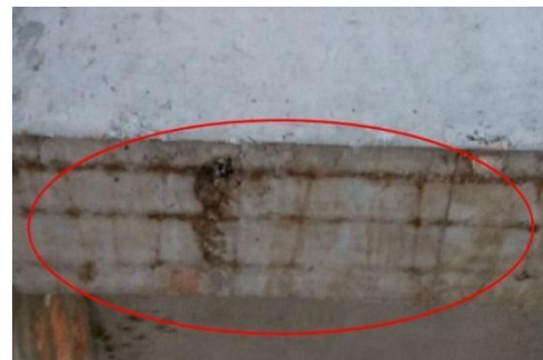
Figure 6. Reinforcements exposed in beam
