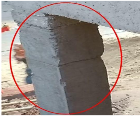
Figure 7. Non-verticality of column
