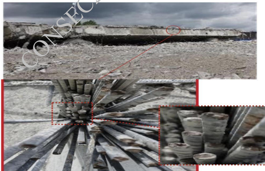
Figure 4. Tensioning wire bundle cracked due to hydrogen-induced stress corrosion cracking in beam 3 bay 2.2 near support C
