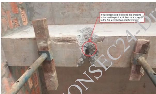
Figure 14. Chipping of Concrete at Beam Marked B2
