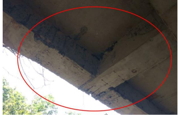
Figure 3. Reinforcements exposed in beam
