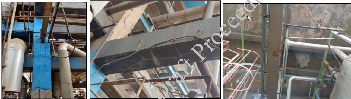
Figure 7. Deteriorated Structural Column, beam & slab before repair
