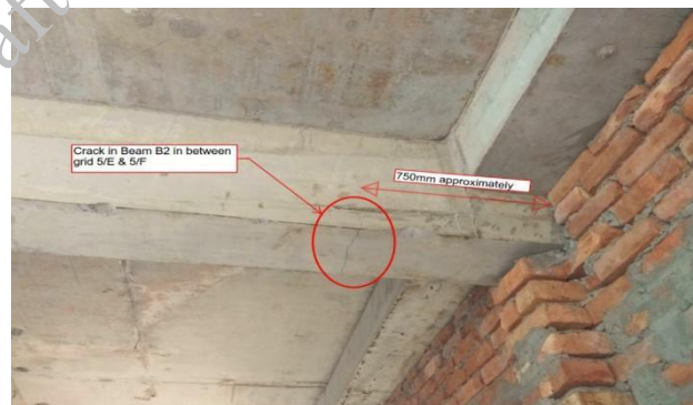
Figure 15. Crack in Beam B2
