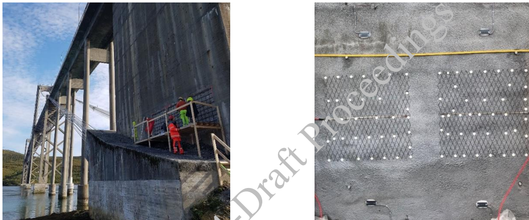
a) Establishing test fields on the northern side of the bridge. b) One test field with titanium mesh and sensors for measuring resistivity, prior to spraying CP-mortar.
