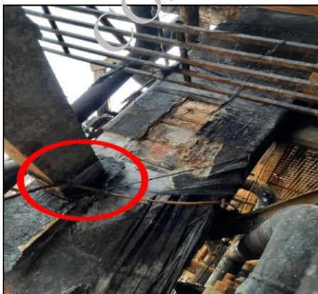
Figure 5. Carbon fiber wrapping burned
