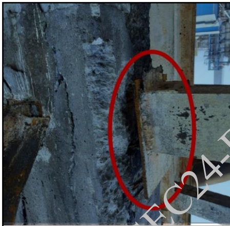
Figure 3: Steel beam came out along with inserts
