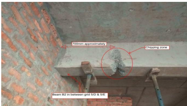
Figure 12. Chipping of Concrete at Beam Marked B2
