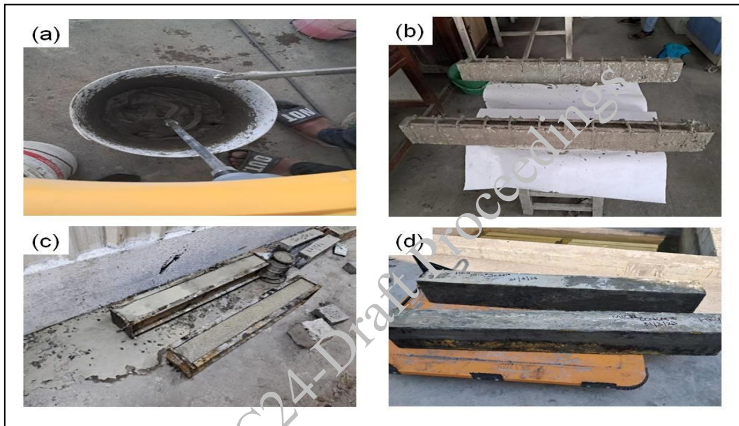
Figure 4. Repairing of beams (a) Mixing of micro concrete (b) View of beams without cover after demoulding (c) Repairing of beams with micro concrete (d) View of beams after repair
