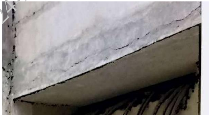
Figure 3. Cracks induced by reinforcement corrosion
