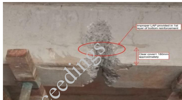
Figure 13. Improper Lapping and Cover
