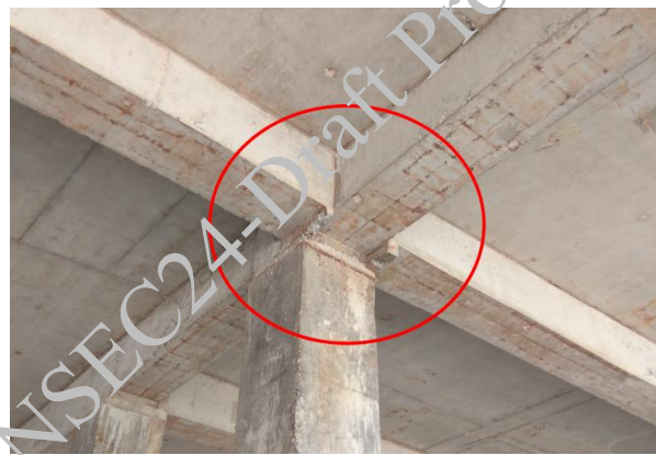
Figure 4. Beams are eccentric at the beam-column junction
