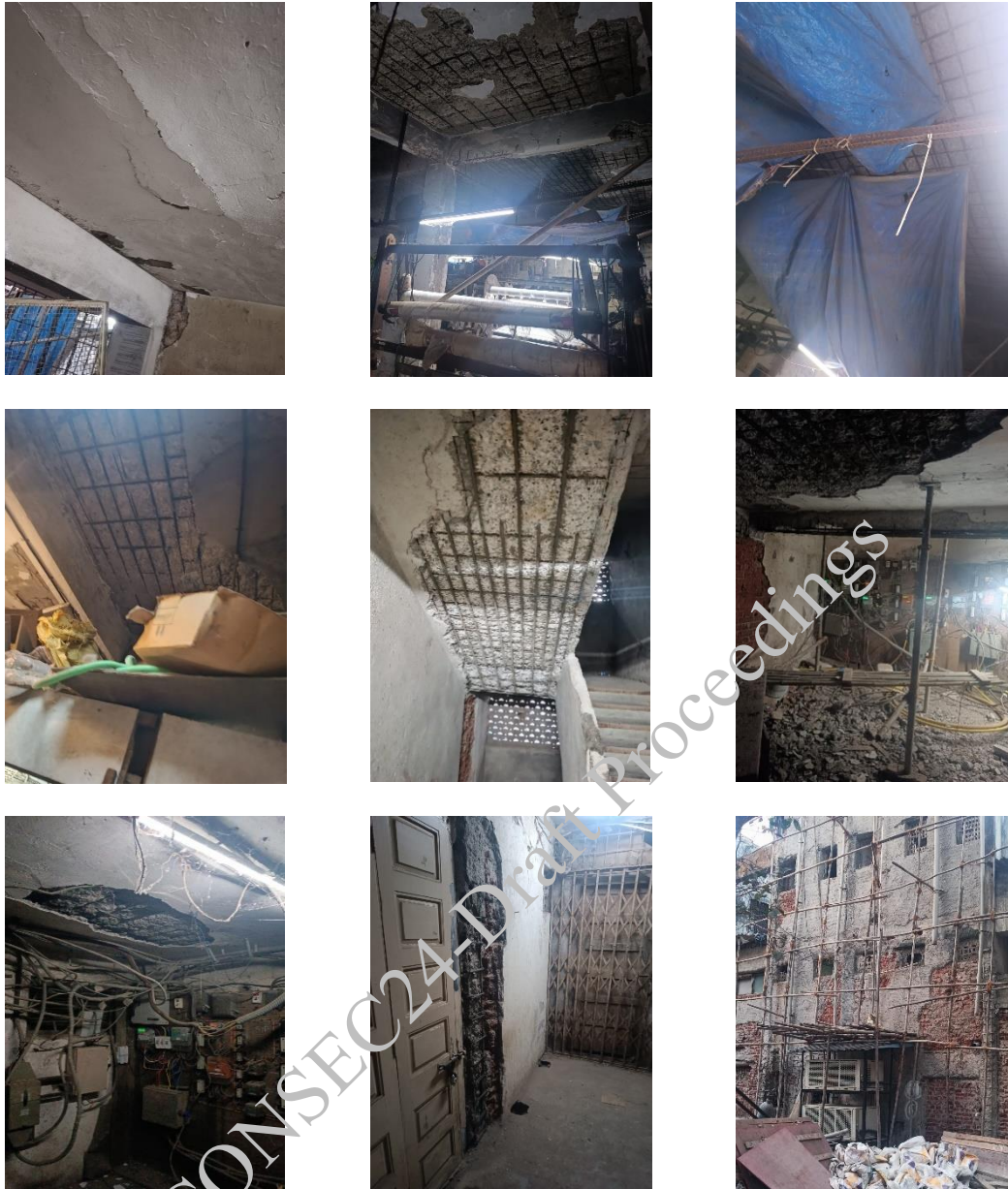
Figure 1. Structural deteriorations observed in the structure
